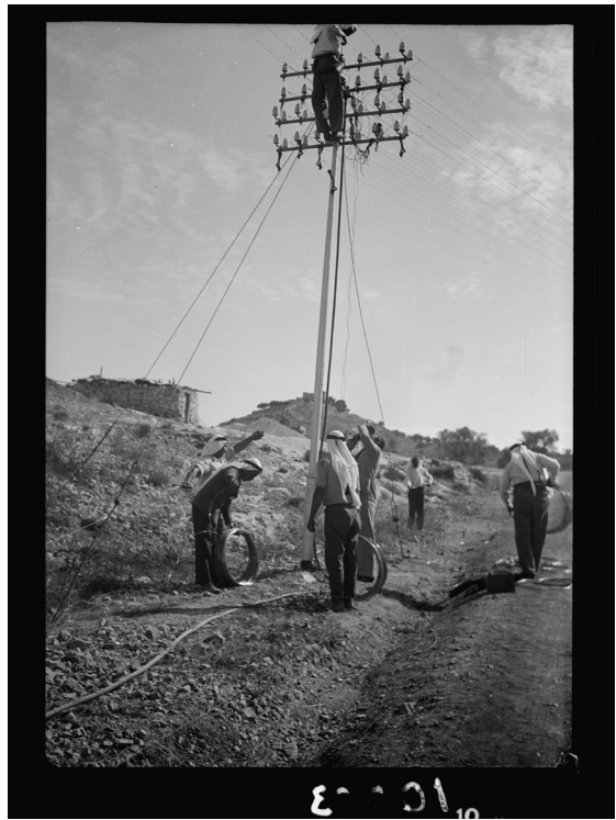
Figure 3. “Repairing telephone lines on Jaffa Road, 31 October 1938.” Matson Photograph Collection, Library of Congress, online at www.loc.gov/pictures/item/mpc2010004369/PP/ (accessed 29 May 2021).
